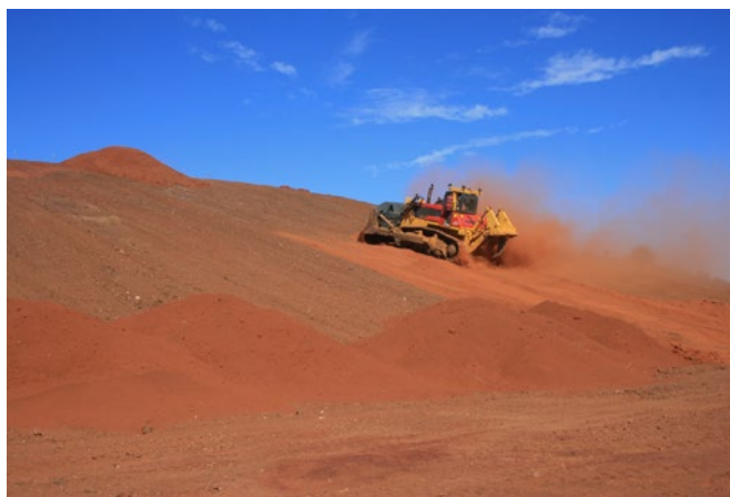
Figure 13. Spreading topsoil on a waste rock dump slope at a mine site. (Photo: L. Commander)
